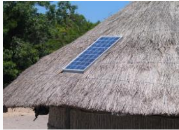
Solar home system
